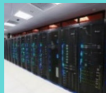
Delta Wujiang IT Data Center LEED V4 ID+C Gold
